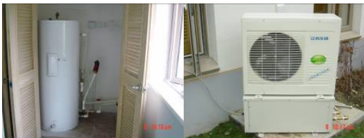
Fig. 16 Photo of air source heat pump water heater
