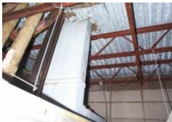
Figure 2: Condensation in the crawl space above the ceiling in bathrooms
