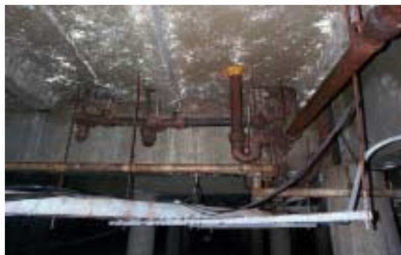
Figure 3: Condensation of the crawl space
