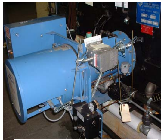
Figure 5 Burner Modulation, showing mechanism of motor, jackshaft, and linkages controlling air damper and oil metering pump
