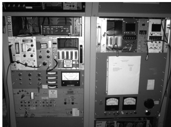
Fig. 11 Control room equipment
