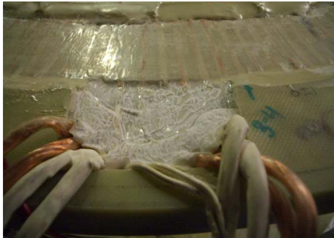
Fig. 9 Wires extending out of wide stator slots
