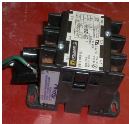
Fig. 12 Relay used to close the circuit
