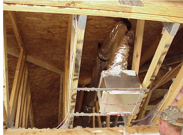
Figure 1 OA Intake Duct in Back Porch
