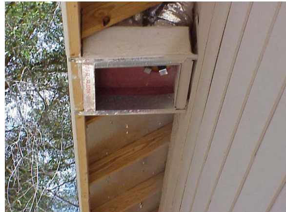
Figure 2 OA Intake Duct in Soffit
