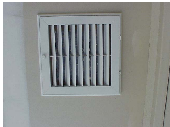
Figure 3 Filter Backed Grill Covering the OA Intake
