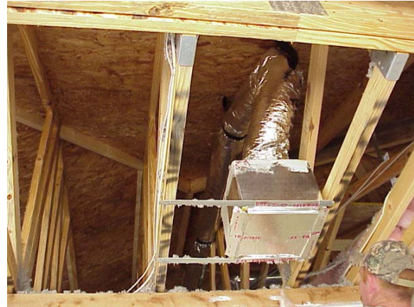
Figure 1 OA Intake Duct in Back Porch
