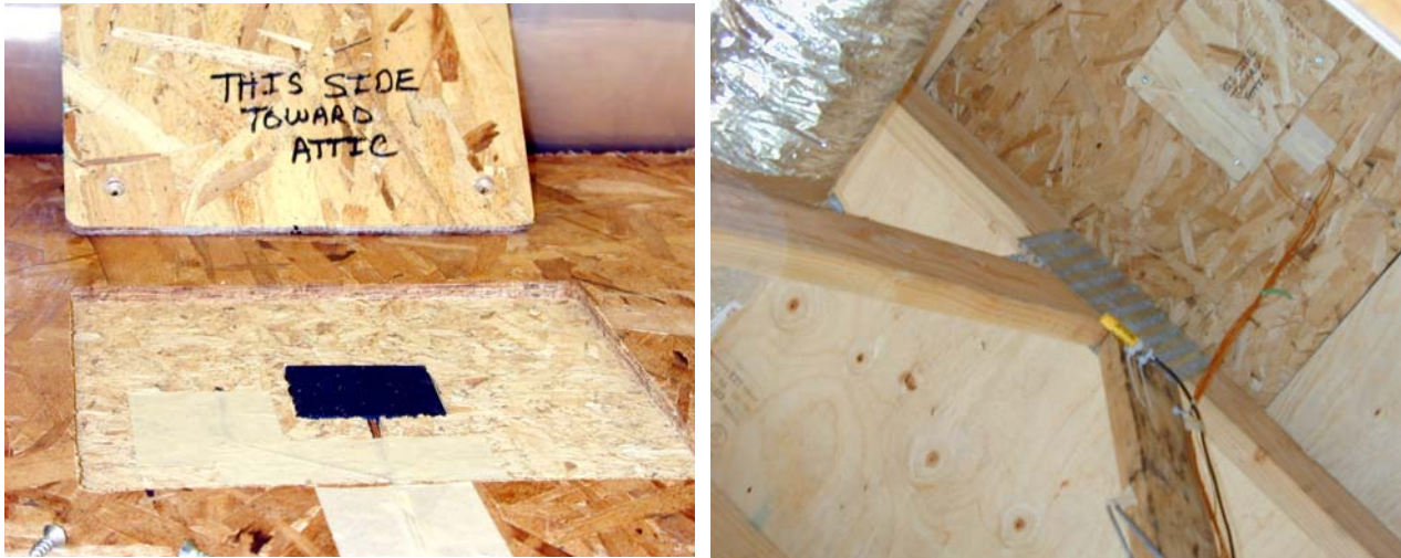
Figure 5. Heat flux transducer embedded in OSB guard and used to measure heat flow crossing roof decks of the demonstration homes with asphalt shingle roofs.
