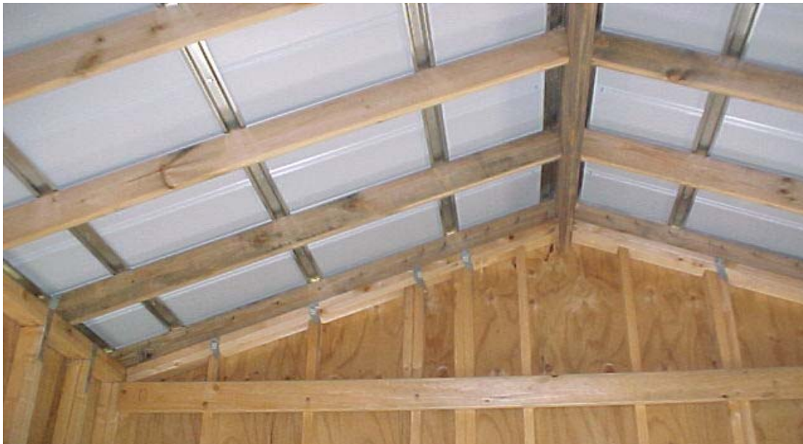
Figure 5: Interior exposed metal roof in attic of NightCool test building
