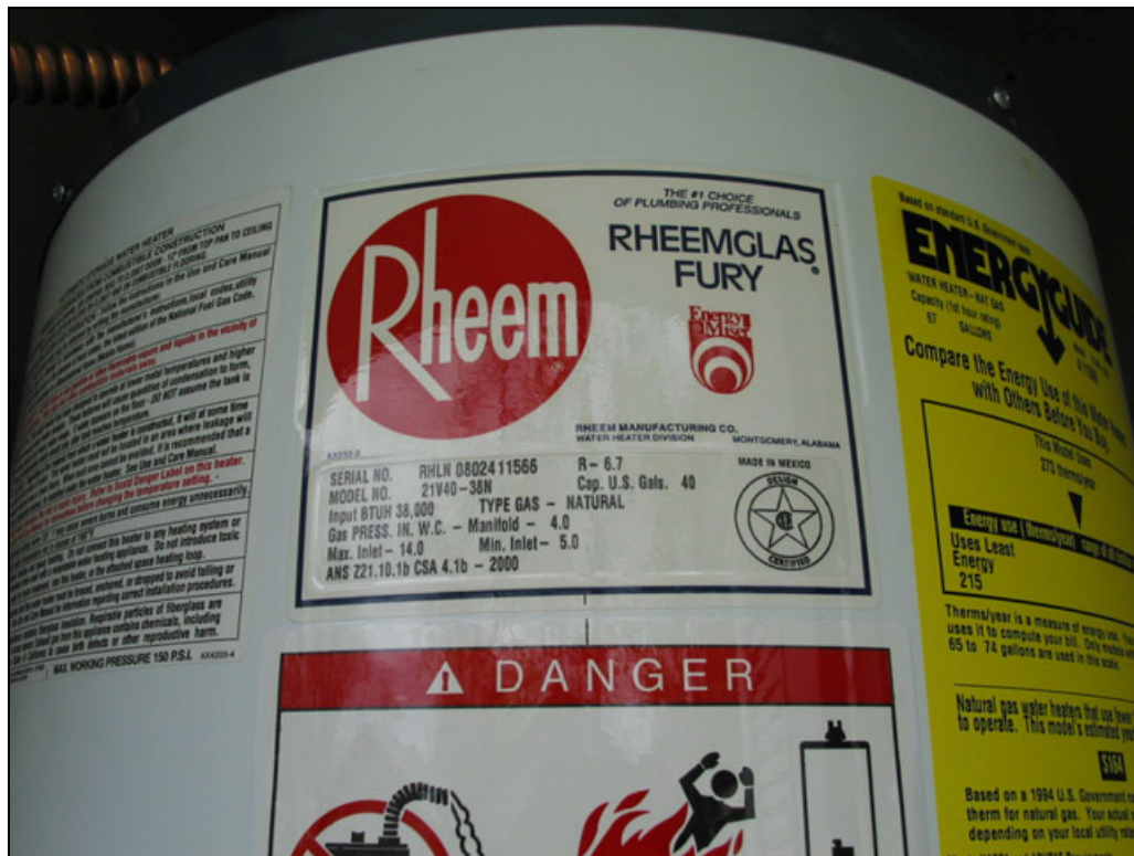
Figure 4.27 – Installed water heater
