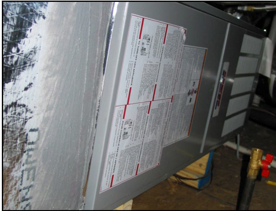
Figure 4.25– Installed furnace in the attic
