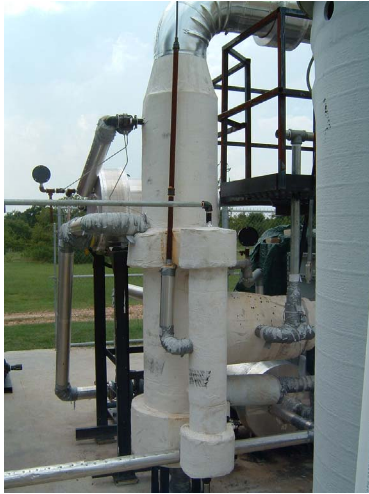
Figure A.31 A closer look at the primary and secondary heat exchangers connected to the jet ejectors, which are used to distill water.
