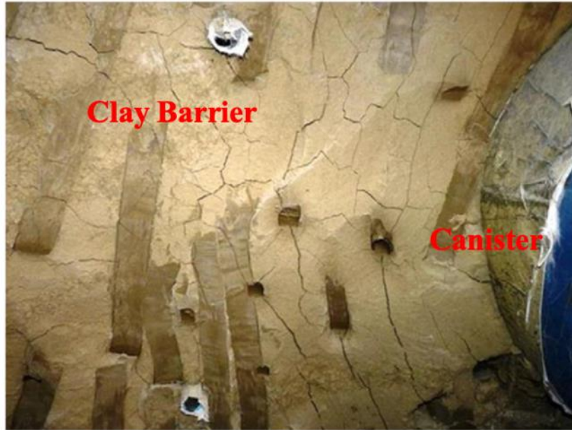
Figure 4.35 Drying cracks observed in a high-level nuclear waste disposal barrier experiment (reprinted from Garcia-Sineriz et al., 2015).
