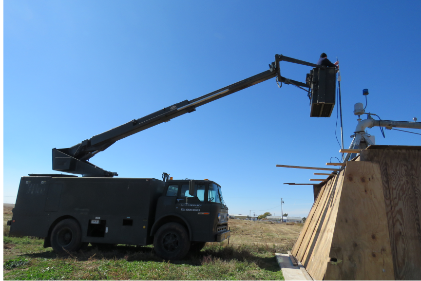
Figure 3.10: Communication system upgrade B, using extension cable to mount antenna high enough to achieve clear line of sight communication.
