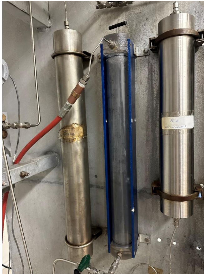
Figure 5 – Water accumulator (left), refill chamber (middle), and acid accumulator (right)
