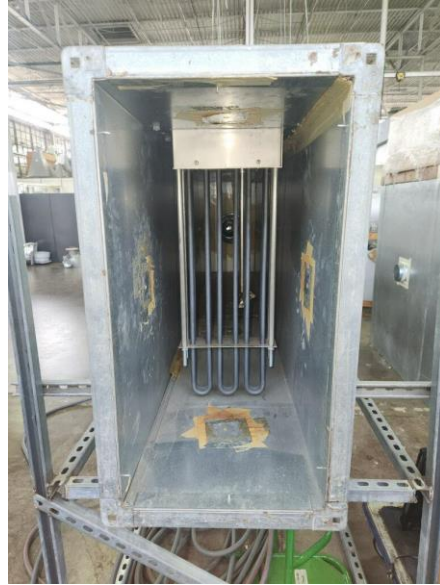
Figure 2.8: Heating element inside of the rectangular intake duct
