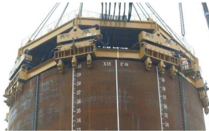
Figure 1.8 Vibratory hammer configuration for project OktaKong. Reprinted from (Van Dorp et al. 2019)
