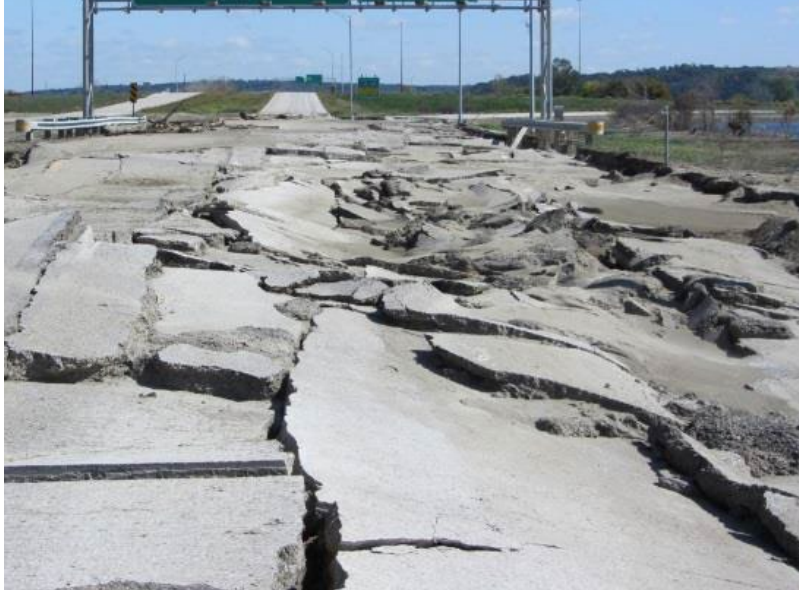
Figure 4. Roadway Damage Due to Flooding in Iowa. Reprinted from [14].
