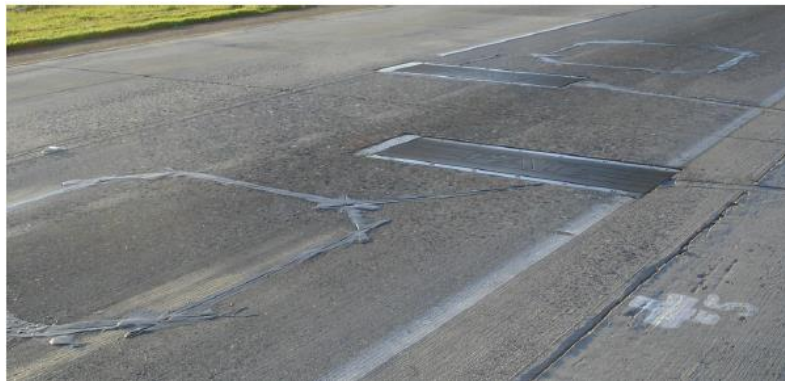
(a) Staggered Bending Plate Installation and Inductive Loops (reprinted from Hallenbeck and Weinblatt 2004)
