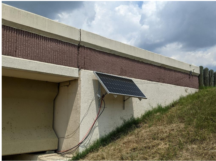
Figure 5.22. Installed Solar Panel (Bridge #2).
