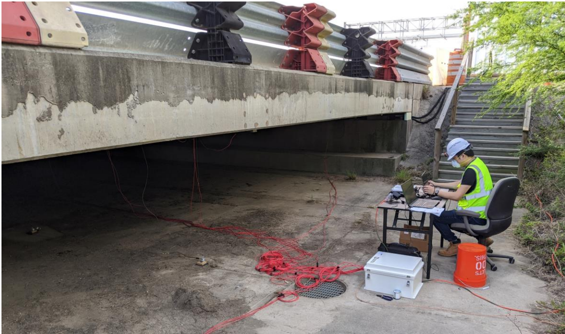
Figure 3.13. Operation of the DAQs.
