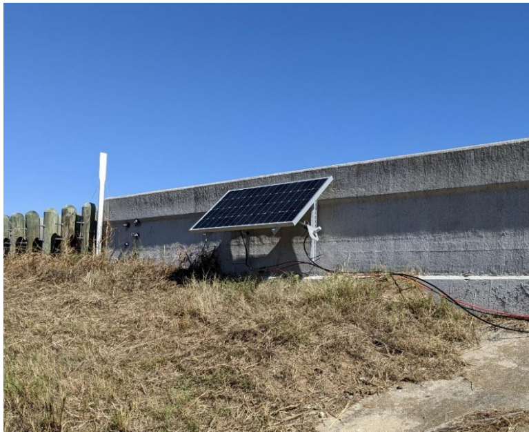
Figure 5.35. Installed Solar Panel (Bridge #3).
