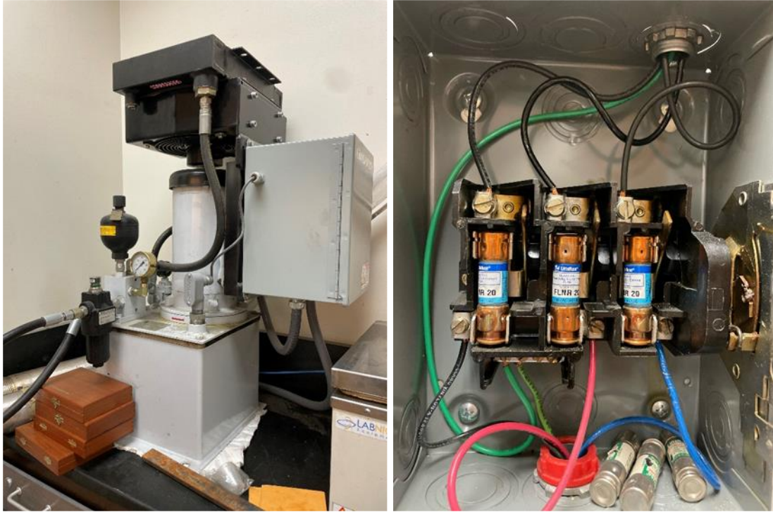
Figure 61. Left - Hydraulic pump that powers the load frame. Right - Fuse box that controls the hydraulic pump.
