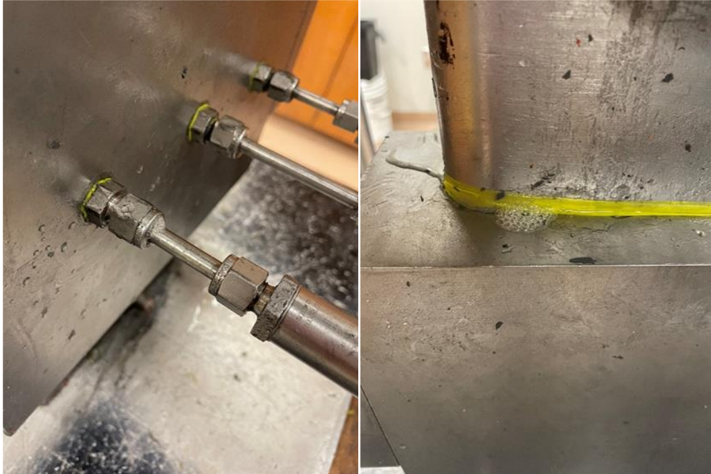
Figure 55. Left - A leak detected on a pressure port. Right - A leak detected on the top piston.
