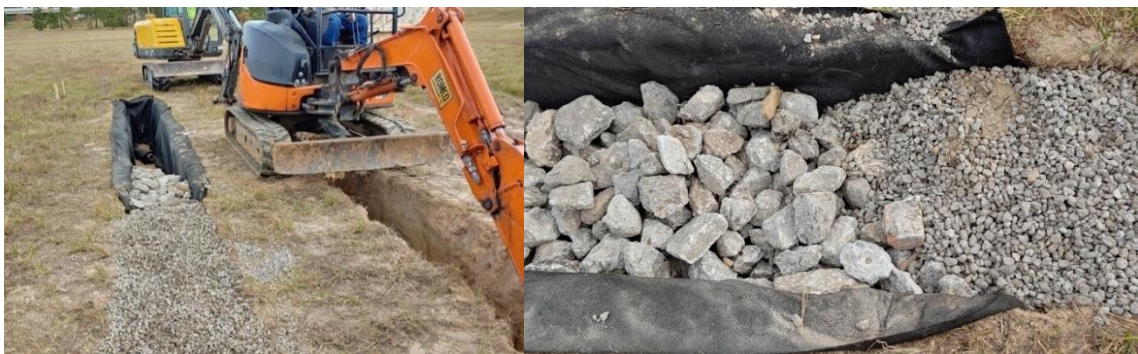
Figure 5. Installation of the trench system (left) highlighting the trench fill and non-woven geotextile fabric (right). Reprinted from Albert et al. (2021).
