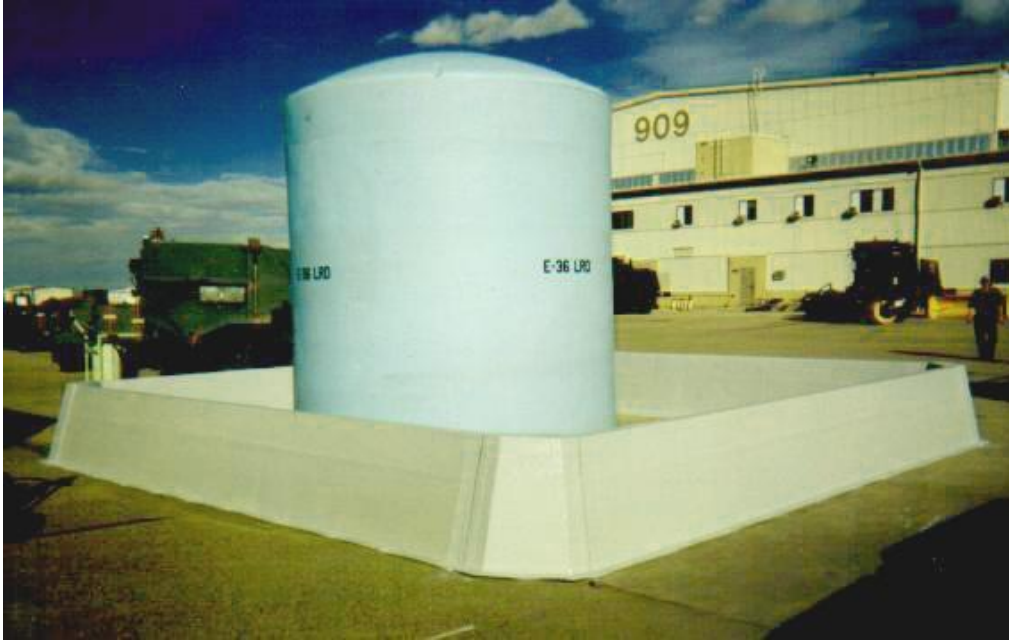
Figure 12: Tank diking (Reprinted from [5]. Parker, T., Shen, R., & Wang, Q., 2022.)
