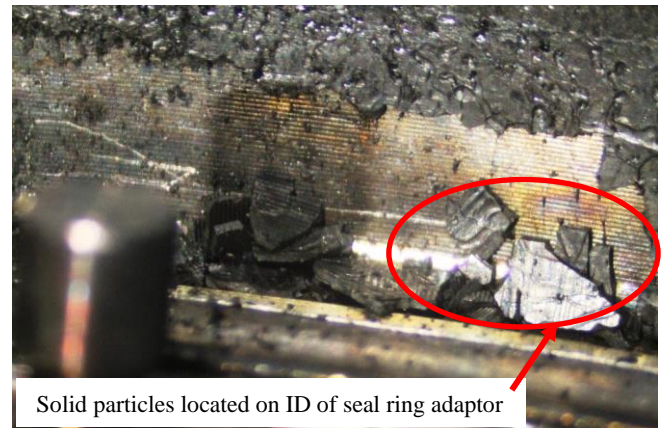
Figure 2: Example of solids build-up on ID of seal ring adaptor, non-interference fitted design
