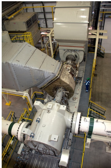
Figure 1: Industrial Gas Turbine powers a gas compressor
