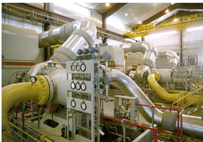
Figure 29: Pipeline Compressor station with 23 compressor trains in parallel
