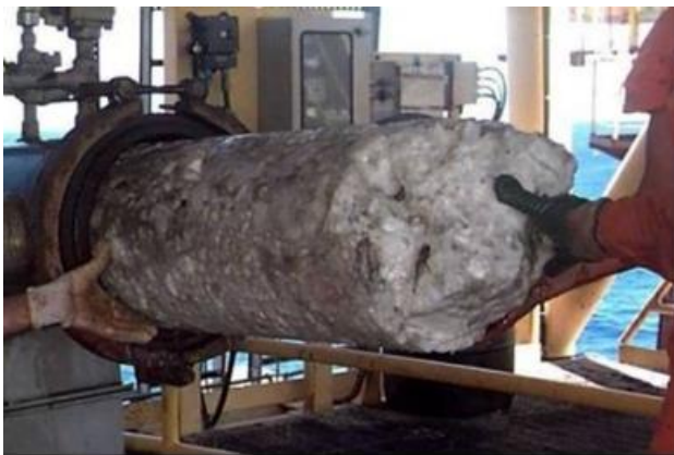
Figure 18: Hydrate formation in natural gas pipeline.
