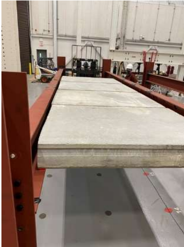
Figure 58: Construction loading of the steel frame – four of five concrete pre-cast panels placed
