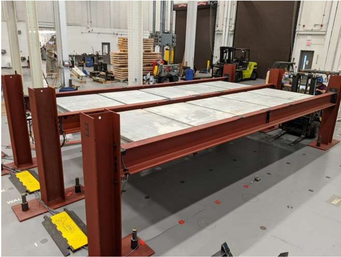
Figure 59: Construction loading of the steel frame – all concrete pre-cast panels installed (image by Matthew Yarnold)
