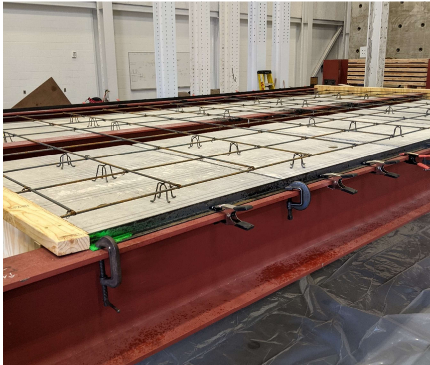
Figure 68: Steel angle concrete form clamped to edge beams (image by Matthew Yarnold)
