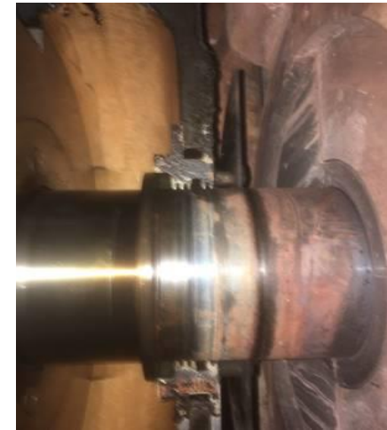
DE oil baffle – exhaust end
