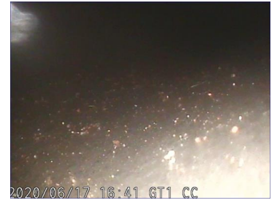
Dirt in fuel gas manifold
