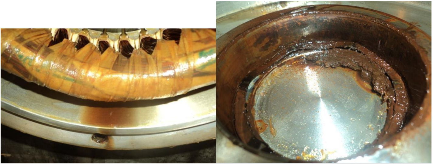
Figure 11: Turning Gear Motor as found damaged on June 6, 2020
