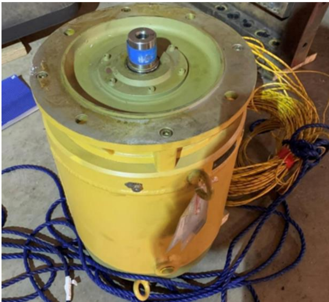
Figure 12: New Turning Gear Motor installed on August 26, 2020
