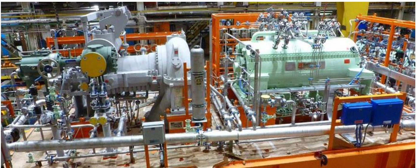
Figure 11: Steam Turbine Driven Wet Gas Coker Compressor
