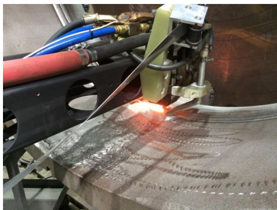
Figure 26 – Electro Slag Welding (ESW) of Strip on Carbon Steel Compressor Flange Face
