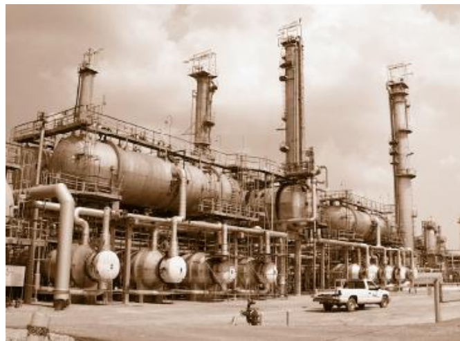
Figure 8: Alkylation Plant (Courtesy of Motiva)
