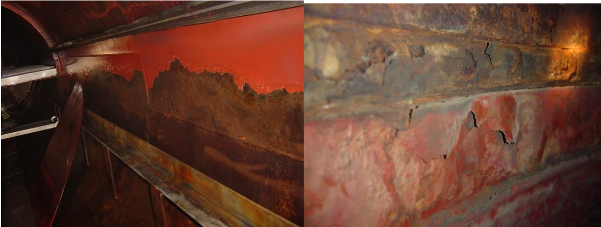
Figure 36: Case Study Three As Found Intercooler Condition
