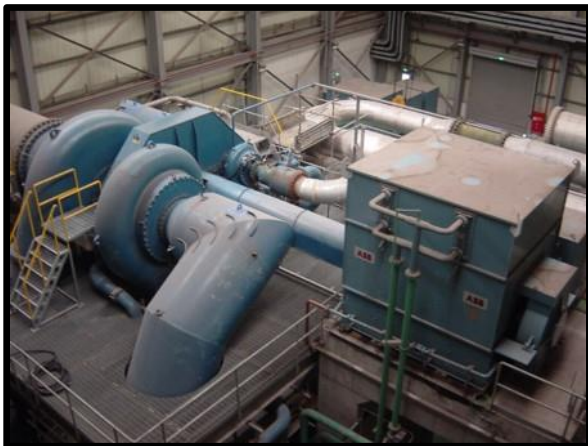
Figure 31: Case Study Three Compressor
