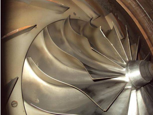
Figure 17: First Stage Blade Failure
