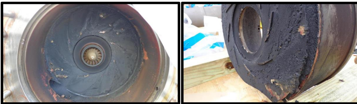
Figure 41: Case Study Four Stage Six Fouling
