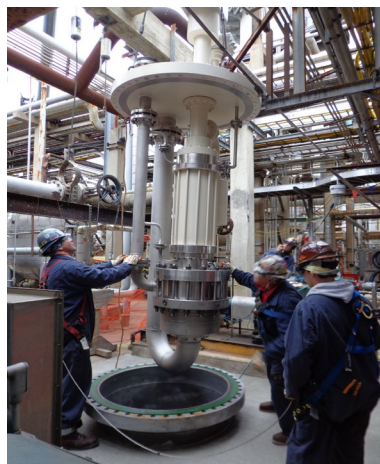
Figure 5 Vertical canned motor pump submerged in Glycol
