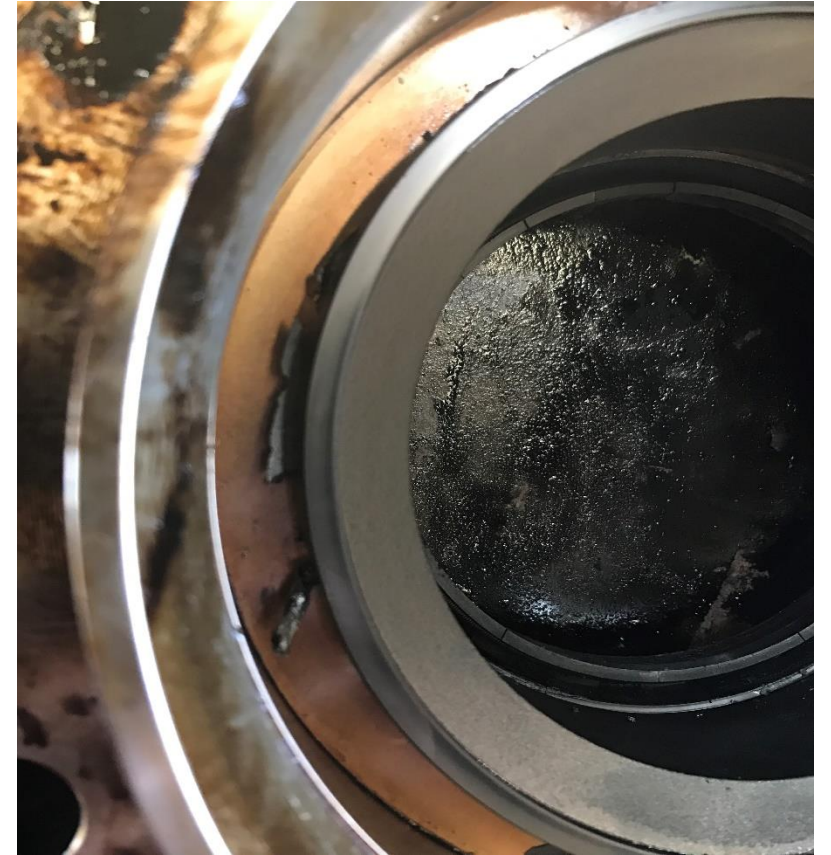
Seal rotating section/face after 18 months operation (partially cleaned) in perfect condition
