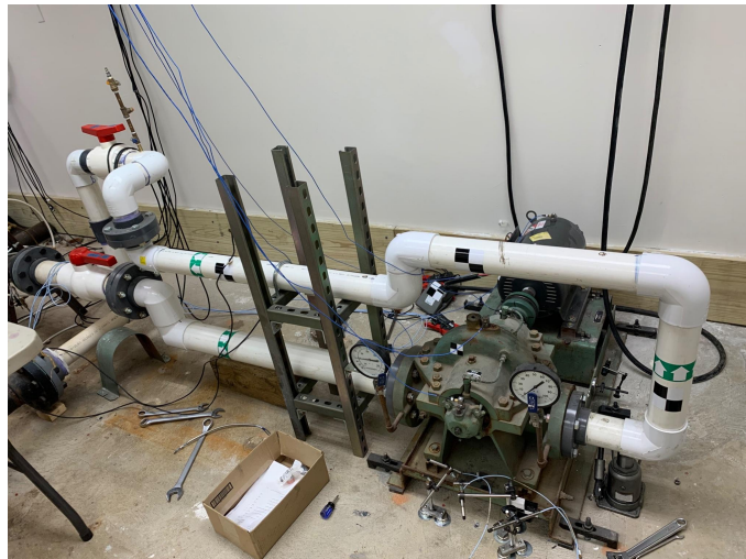
Figure 3(a). Motor Pump used for the experiment
