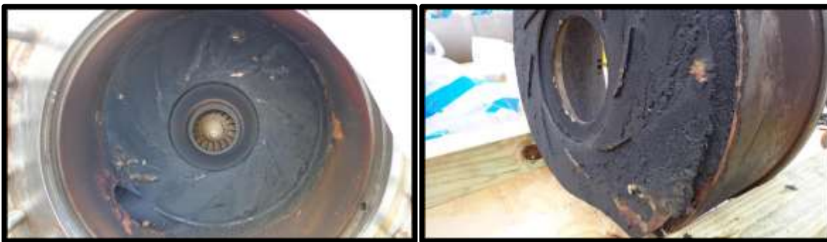
Figure 41: Case Study Four Stage Six Fouling
