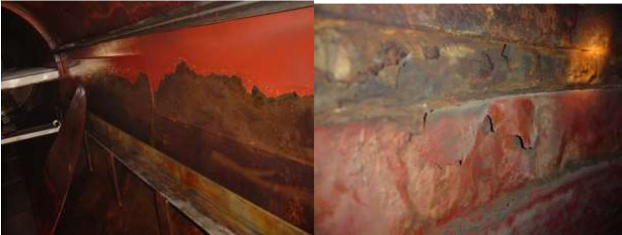
Figure 36: Case Study Three As Found Intercooler Condition
