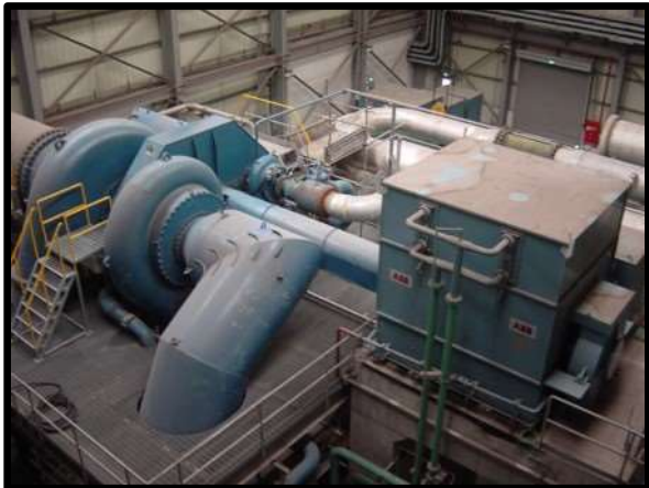
Figure 31: Case Study Three Compressor
