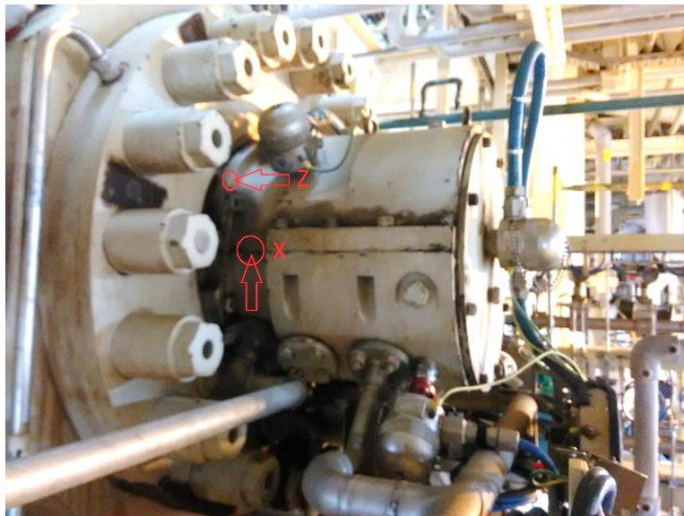
Figure 3 – Offline Bearing Housing Measurements
