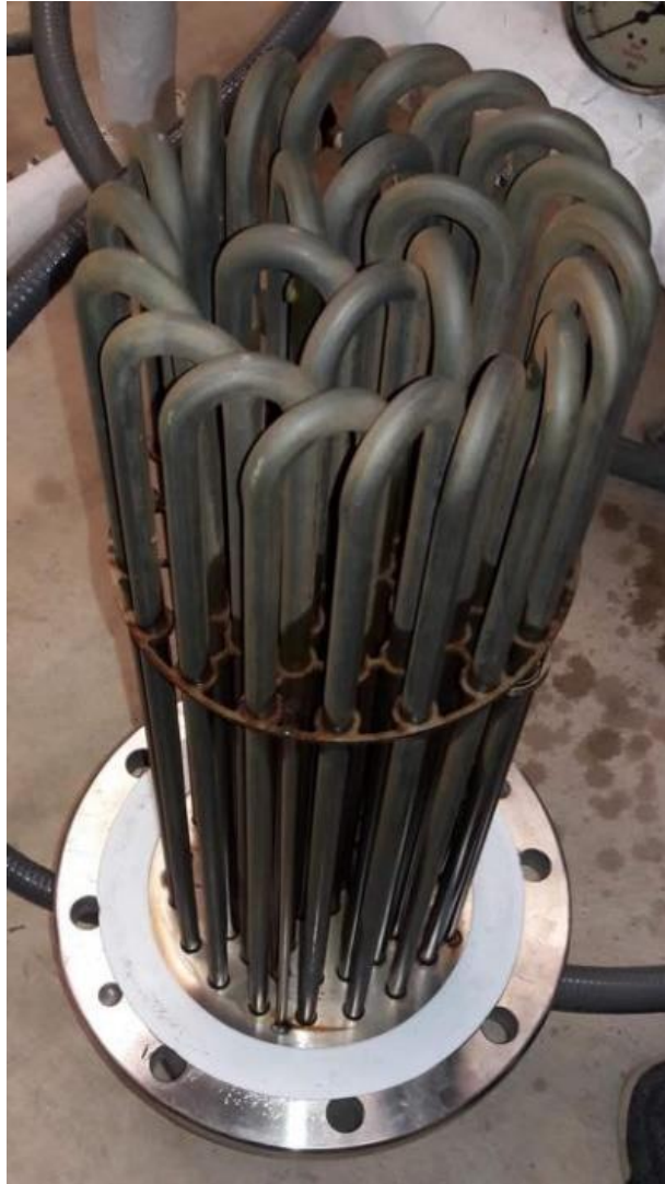
Figure 3.6 The u-tube shaped immersion heaters for the Steam Generator
