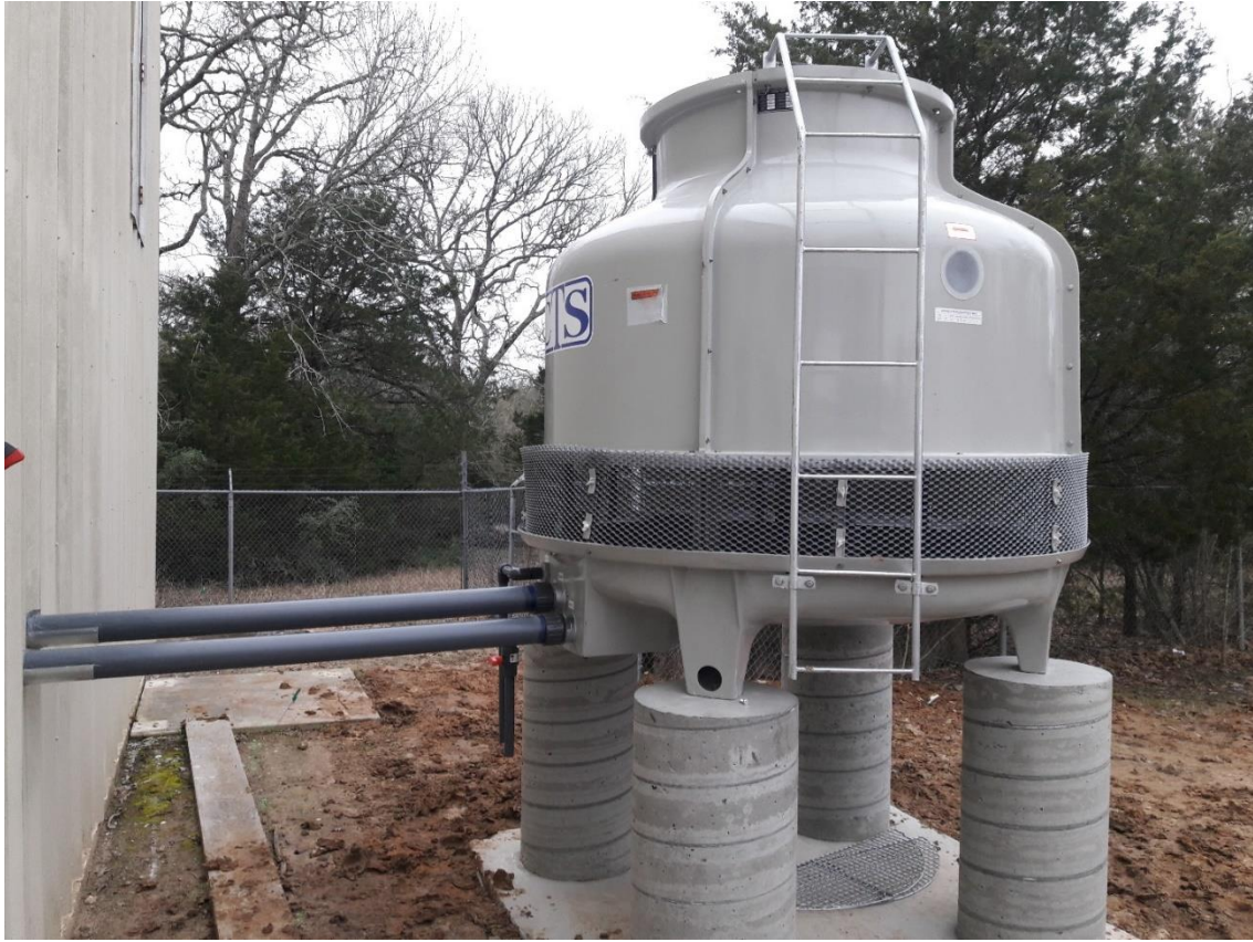
Figure 4.17 NHTS Cooling Tower
