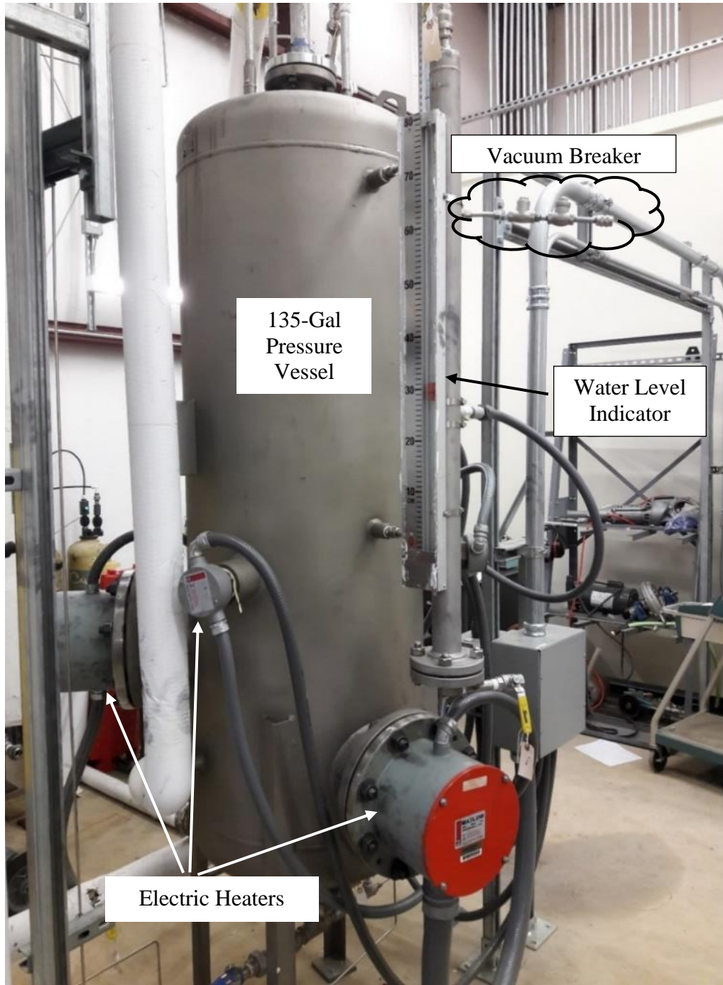
Figure 3.3 Steam Generator with visual water level indicator
