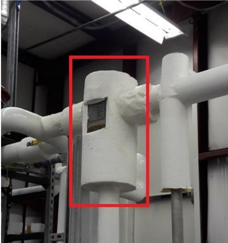
Figure 3.7 Separator downstream of the steam generator outlet
