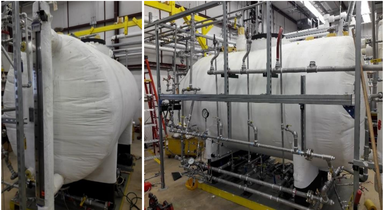
Figure 3.11 Suppression Pool front side (left) and wide view (right)
