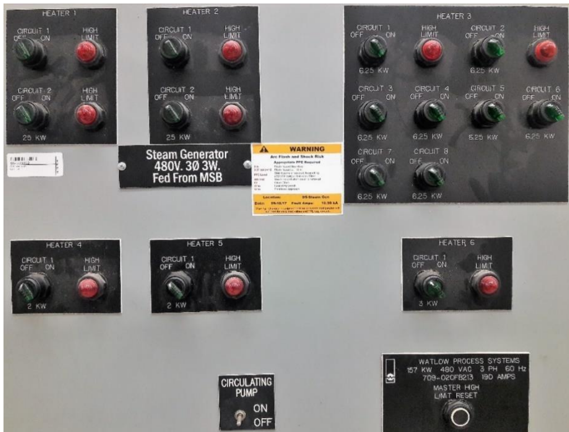
Figure 3.5 Heater control panel
