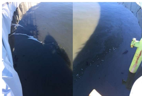
Figure 34: Aboveground storage tank (AST)
