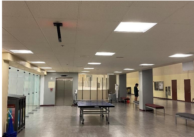
Figure 5.35: Fluorescent tubes in common area (at 5 ft. distance)
