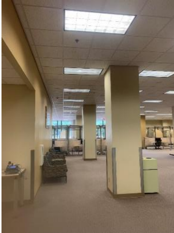
Figure 5.20: Fluorescent lighting on first floor: 12 ft. height
