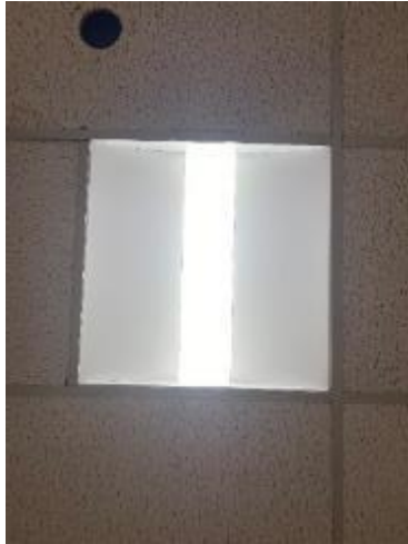
Figure 5.13: Representative LED tube (first floor)
