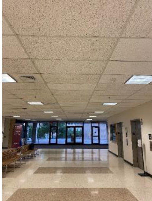
Figure 5.15: Fluorescent lights (5 ft. height)
