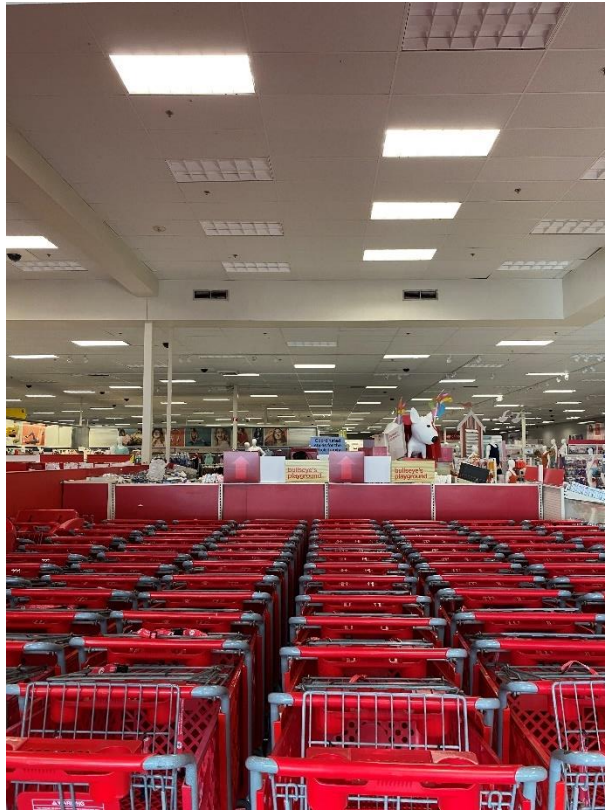
Figure 5.52: LED lights at Target Mall (at 12 ft.)
