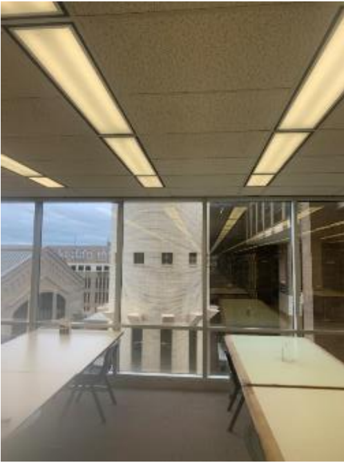
Figure 5.22: Fluorescent lighting: 5 ft. height (presence of ambient light)
