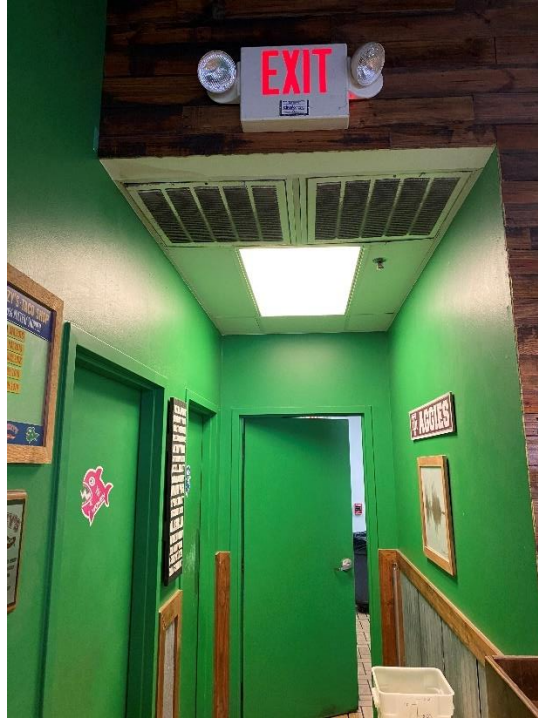
Figure 5.42: Fluorescent tube near restroom (3 ft. distance)
