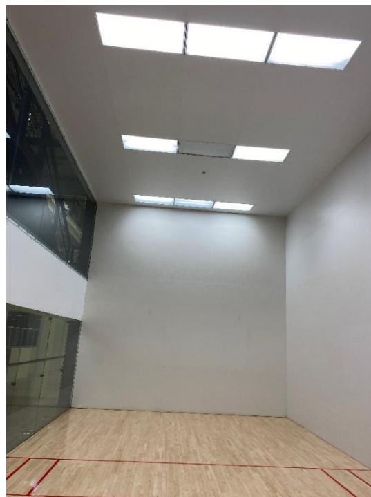
Figure 5.36: Fluorescent tubes in racket ball room (at 15 ft. distance)
