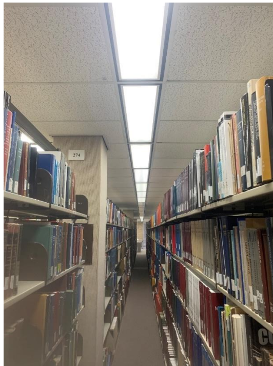
Figure 5.21: LED lighting in the aisles of third floor: 5 ft. height
