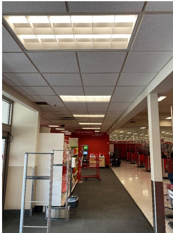
Figure 5.51:LED lights at Target Mall (at 4 ft.)
