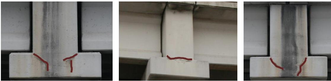
Figure 1-2. Observed Cracks on In-Service Inverted-T Bent Caps (US 290 in Austin).
