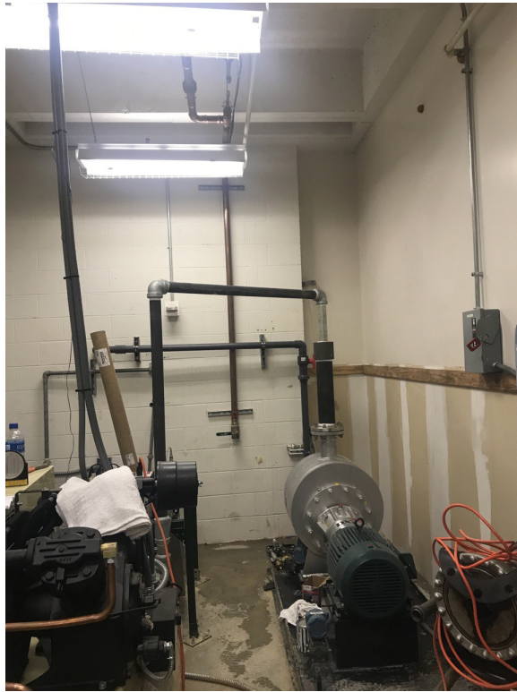
Figure 3-7—Multiphase Twin Screw Bornemann Pump and Supply Pipes
