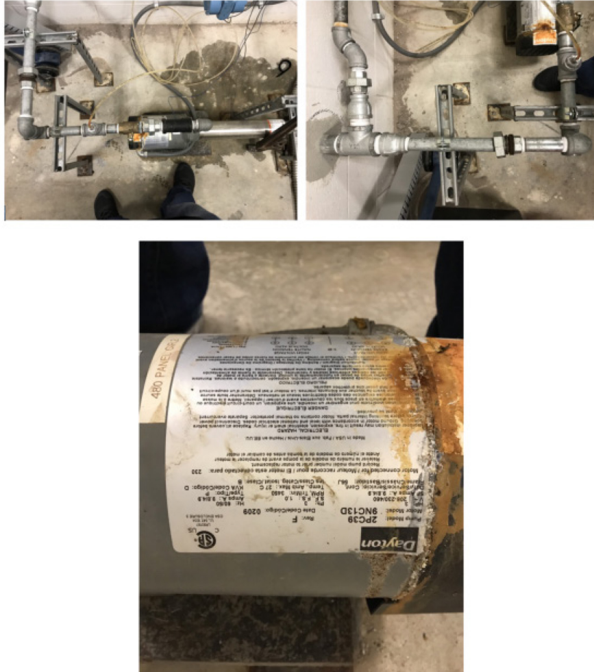
Figure 3-4—Damaged Boost Pump
