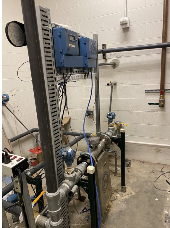
Figure 3-6—1-1/2-in MicroMotion Mass Flow Meter (Bottom) and Flow Transmitters (Top)
