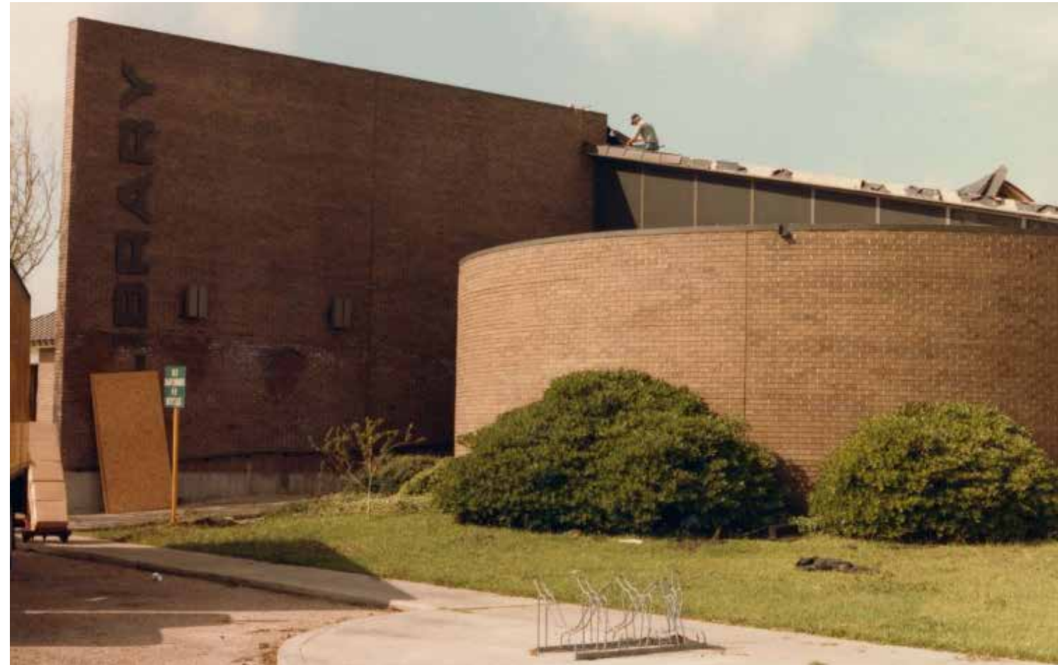
1983 - NORTH EASTERN VIEW OF LIBRARY - ROOF WAS DAMAGED BY HURRICANE ALICIA
