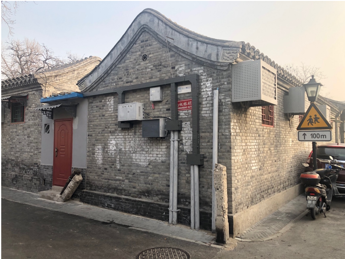
Figure 12. Re-arranged and covered electronic wires on the side wall of a courtyard house in Dongsi Liutiao. Photo by the author.
