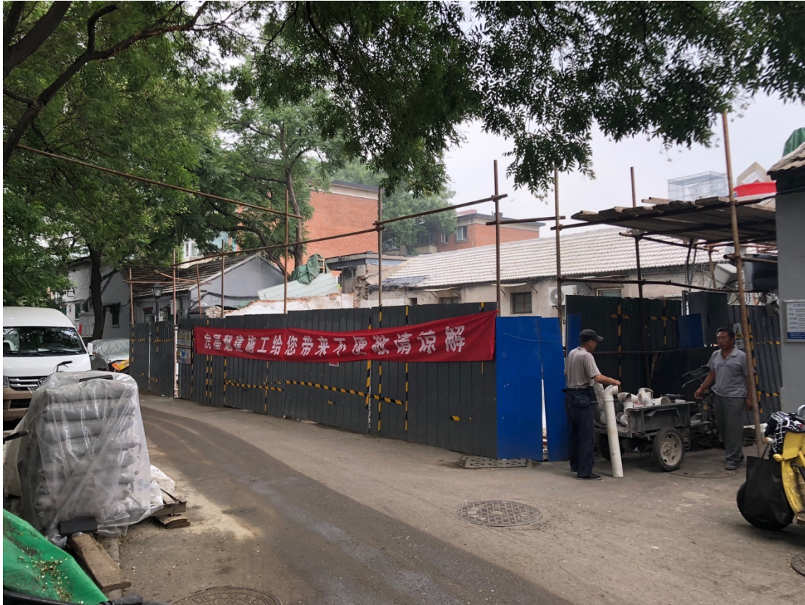
Figure 13. A covered construction site in Dongsì Qítiao with a “excuse our mess” banner. Construction or renovation plan needed to be reported to the neighborhood committee and the residents are responsible to arrange labor or service to remove any construction waste from the site. Photo by the author.
