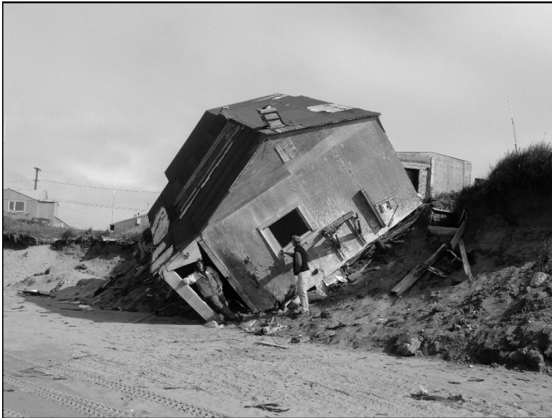
Figure 15 House tipping in Shishmaref, Alaska. (Photo by J. Giardino, 2006). Reprinted with permission from Aguilar et al., 2020.
