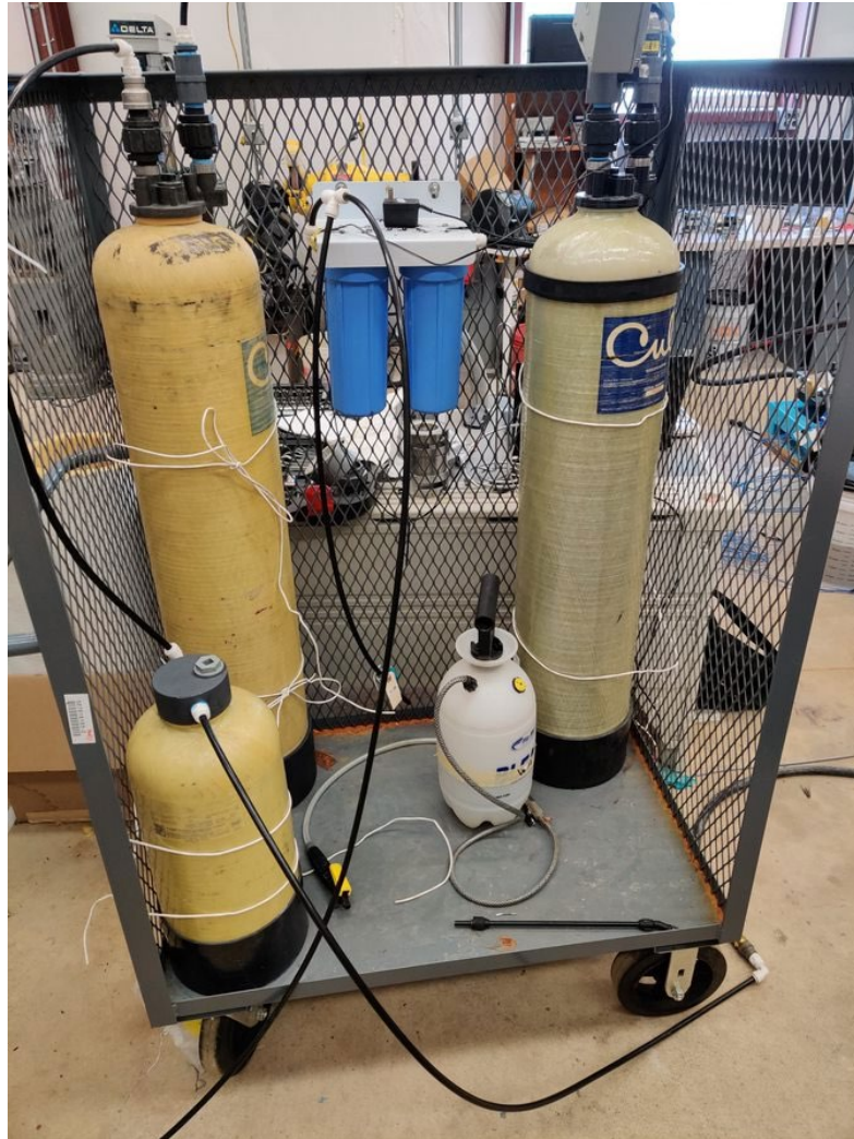
Figure 3.2. Culligan® DI water filtration system on mobile cart.
