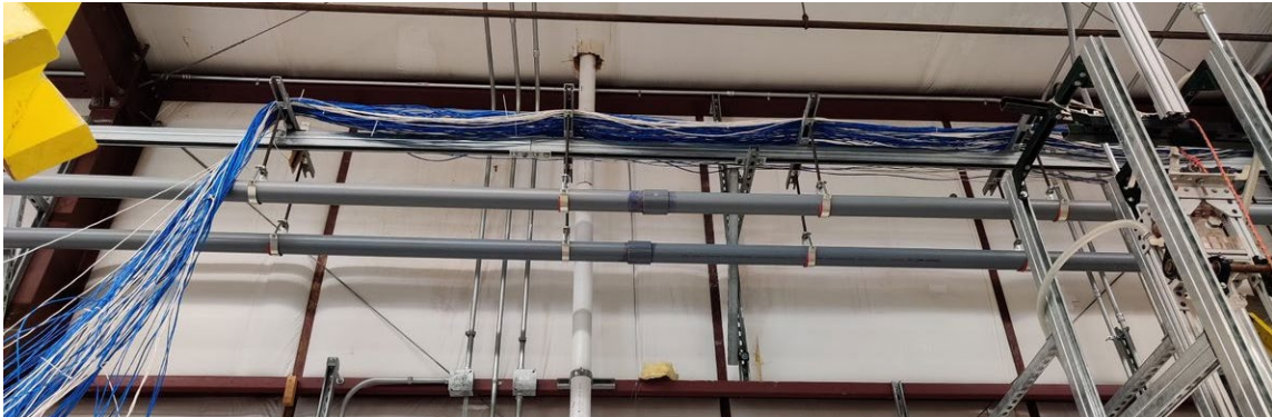
Figure 3.41. HRS elevated piping section #4. Blue and White instrumentation wires run along the top of the pipe support structure.
