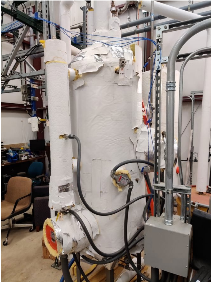
Figure 3.6. Steam generator vessel.
