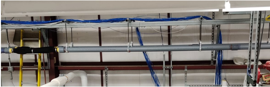
Figure 3.39. HRS elevated piping section #2.
