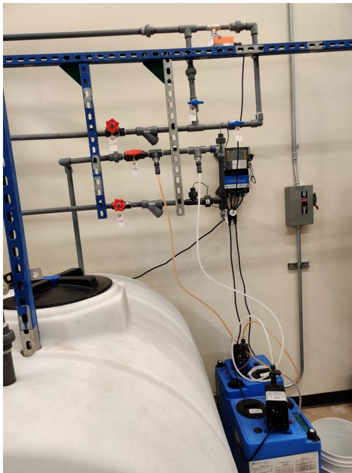
Figure 3.26. HRS Water Treatment System.
