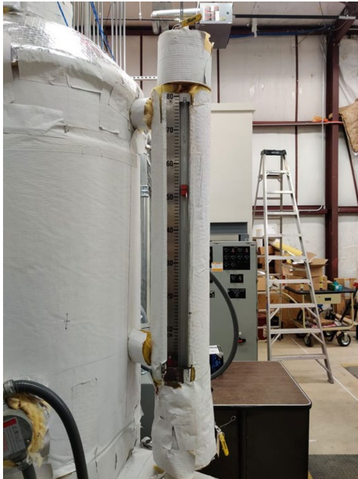
Figure 3.10. Steam generator water level indicator.
