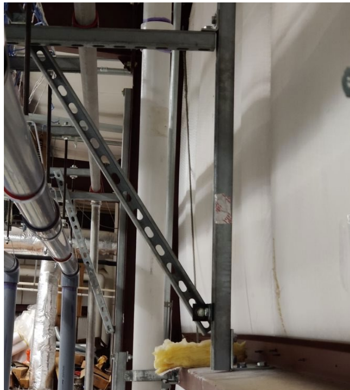
Figure 3.37. Triangular supports bear the weight of the main support structure and fix it to the wall.
