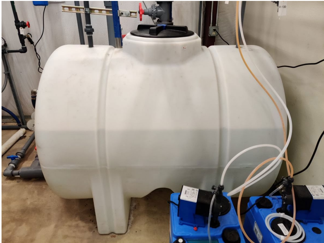
Figure 3.23. Photo of HRS Storage Tank as installed in facility.
