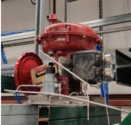
Figure 3.12. Masoneilan 21124 Top-Guided Globe Valve, used to control steam flow rate.
