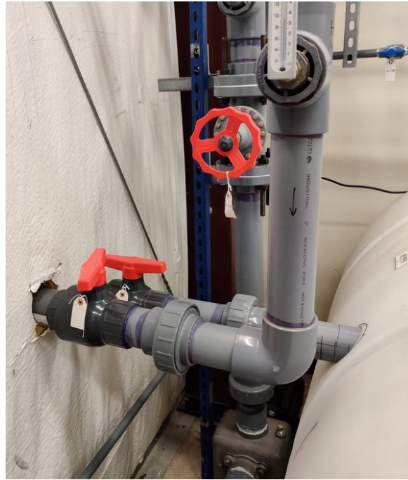
Figure 3.35. 3-inch pipes penetrating the wall route to the inlet and outlet of the HRS cooling tower. 3-inch pipe extending upward from the HRS secondary-side pump goes to the HRS heat exchanger and water treatment systems. Red globe valve controls the flow rate through the HRS piping system.
