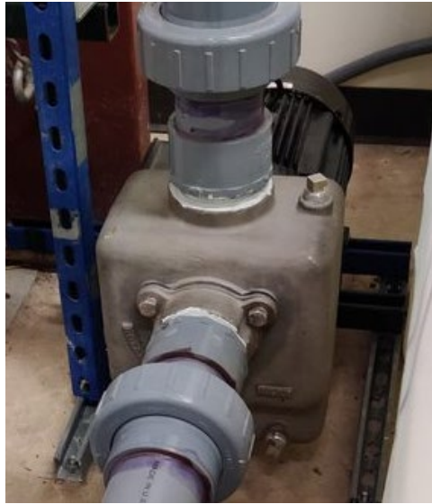
Figure 3.29. HRS secondary-side coolant pump. Dayton 12N813 Self-Priming Centrifugal Pump.
