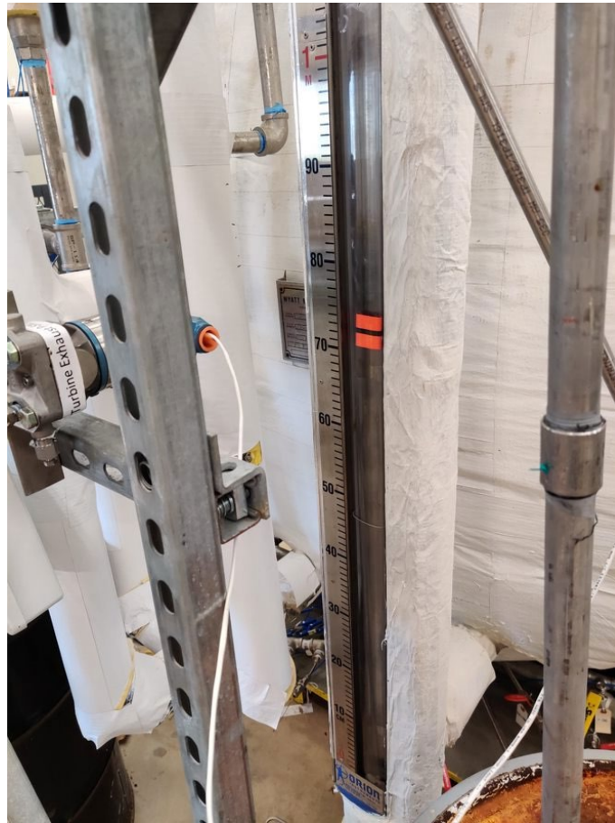
Figure 3.5. Suppression chamber analog water level meter.
