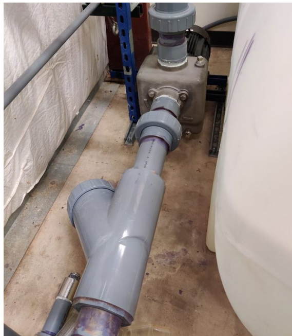
Figure 3.34. HRS secondary-side piping. Water passes through the Y-strainer before entering the pump.
