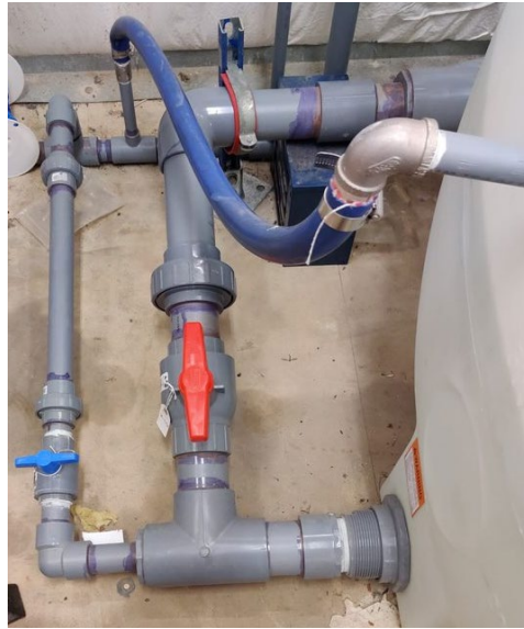
Figure 3.33. HRS Tank outlet. 3-inch pipe with red ball valve leads to HRS secondary pump. 1.5-inch pipe with blue ball valve leads to floor drain.
