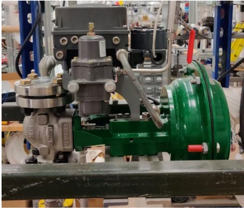
Figure 3.14. Fisher D041TV1 DN25 GX air-to-open globe valve. Used to control the flowrate of water returning to the steam generator.
