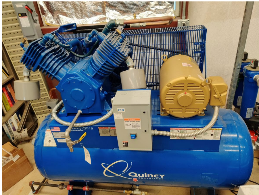
Figure 3.49. Quincy Air Compressor.
