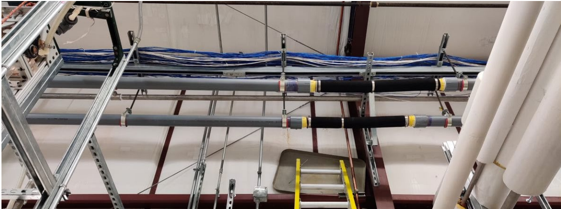
Figure 3.40. HRS elevated piping section #3. Black flexible hose helps to account for thermal expansion.
