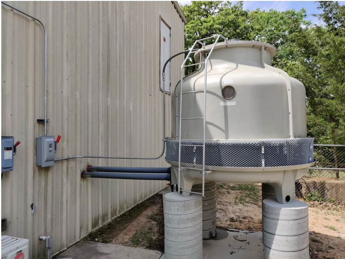
Figure 3.22. HRS Cooling Tower.
