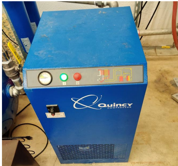
Figure 3.50. Quincy Compressed Air Dryer.
