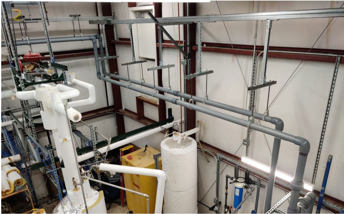
Figure 3.38. HRS elevated piping section #1.
