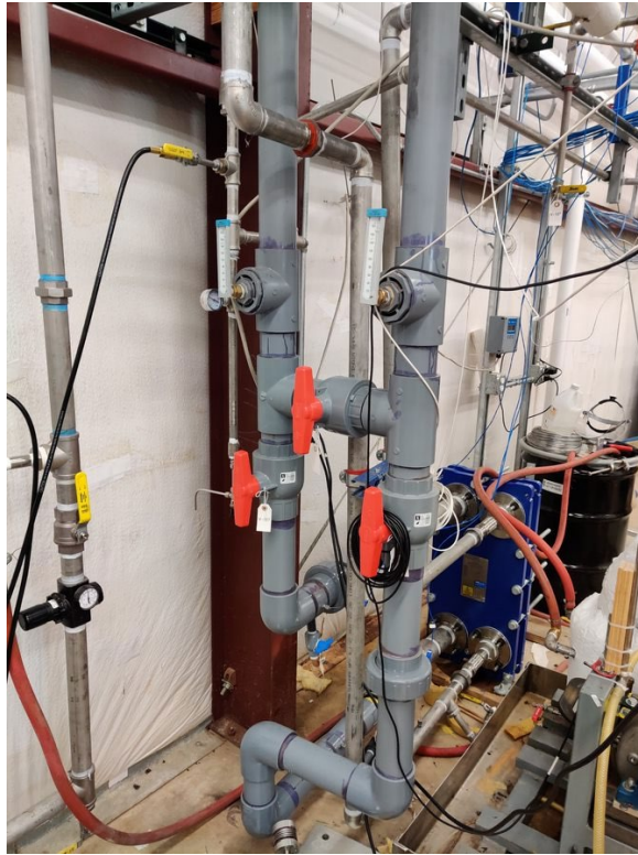
Figure 3.43. HRS piping. Red ball valves allow for heat exchanger bypass.
