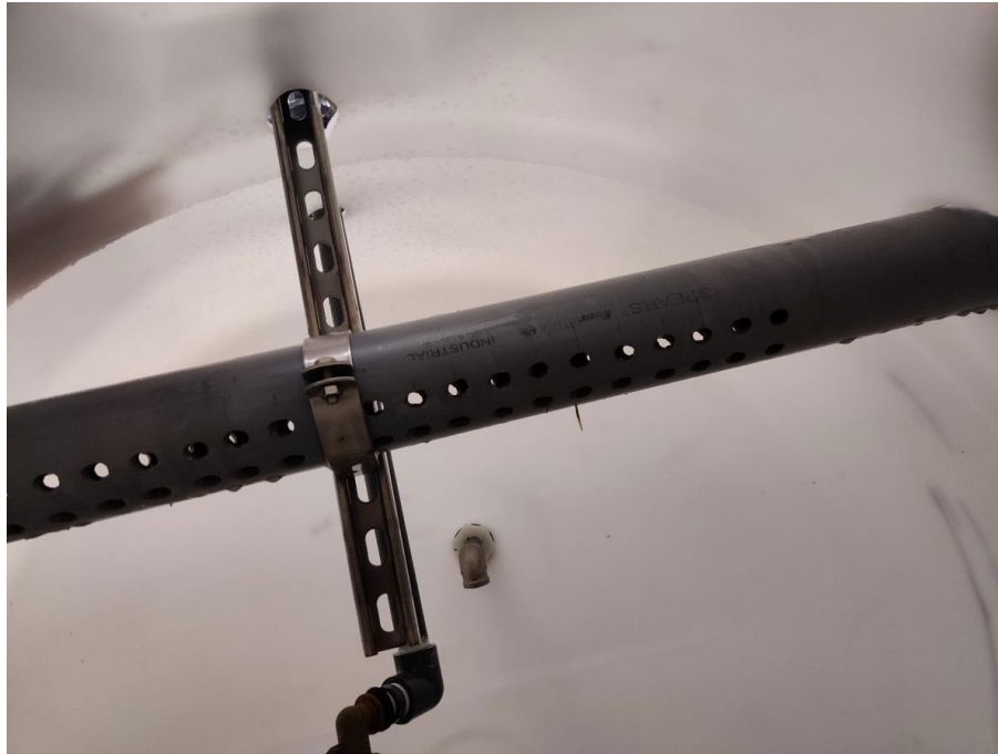
Figure 3.25. Water return line from HRS cooling tower supported by stainless steel channel strut.
