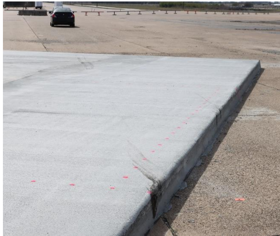
Figure 3.11 Tire traces on the sidewalk after the test completion
