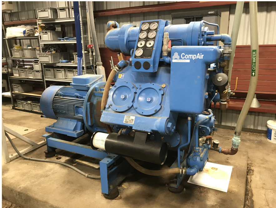
Figure 2.1: One of the two (soon to be three) CompAir 5442 compressors.
