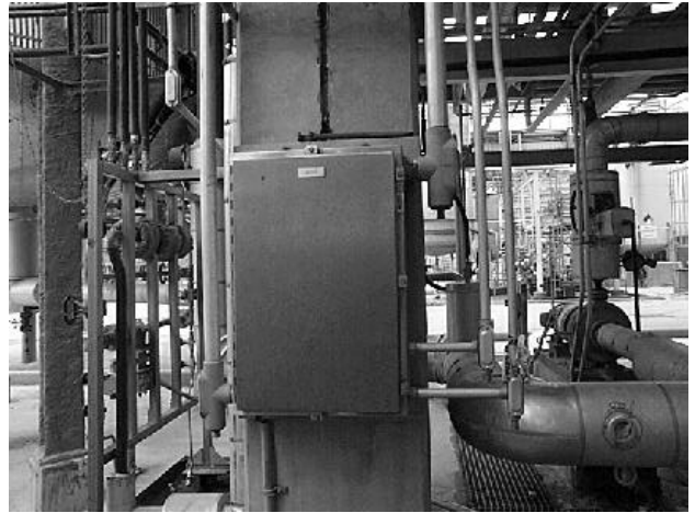
Figure 15: Conduit Box Prone to Water Entry
