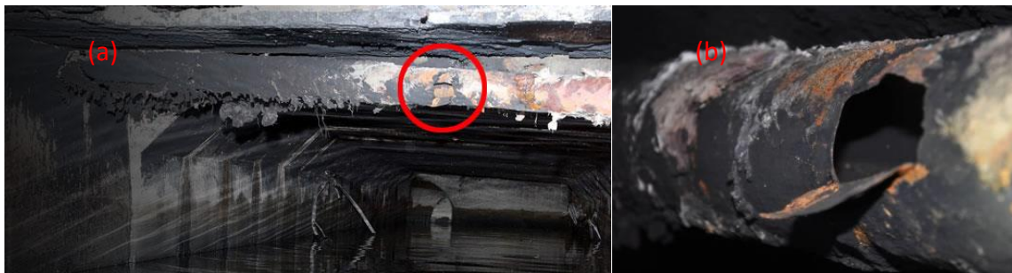
Figure 5: Photos of (a) the storm water trench, the 4-in propylene pipeline and the break, (b) close view of the break opening.
