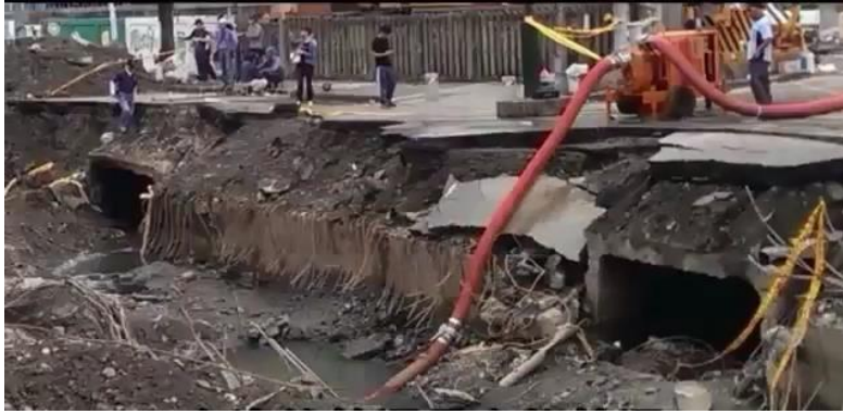
Figure 7: Photo of the storm water trench branches, the left one housed the pipelines and the right one was sealed in the other end with a total length about 7 m.
